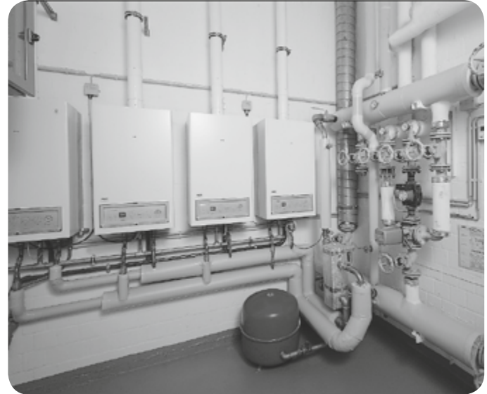
Heating boilers connected in cascade
